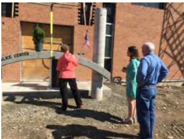
Cheryl Kurosky of the BCC Foundation Board signs the last piece of steel erected as part of the Calice Center.
