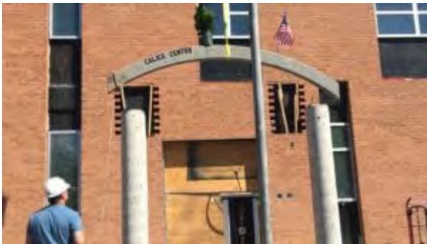
The last piece of steel is erected as part of the Calice Center’s south entrance canopy.
