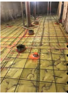
Concrete basement floor ready to be poured in the vicinity of the Beverage Lab in the Culinary & Event Center
